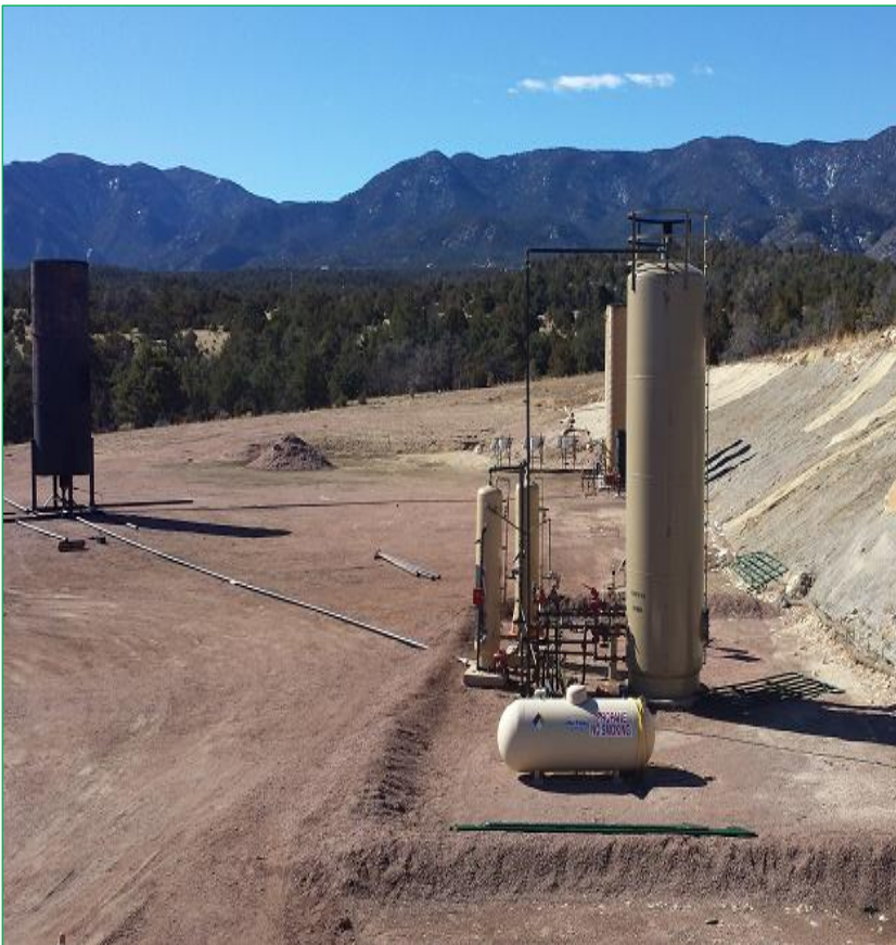
Figure 2: Oil and gas separators installed for higher gas volumes
